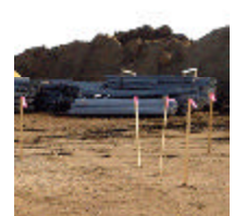
Lighting Materials - Valley Stadium
