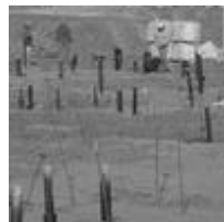
Plumbing Stacks - Valley Stadium
