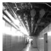
Main Corridor Piping - Stilwell
